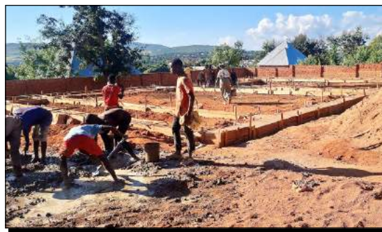
Foundations being constructed for a new apprenticeship training center. More info in our next newsletter.
